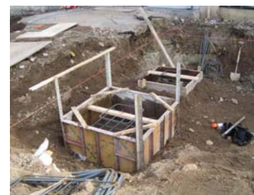
The foundation for the pillars which will hold up the overhang at the front door.
