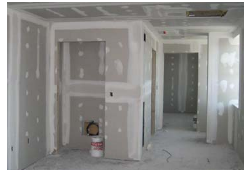
Now the kitchen cabinets are in place on the third floor and the finished sheetrock is ready for a first coat of paint.
